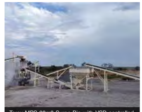
Terex MPS 20m3 Surge Bin with VSD controlled Pan Feeder and Conveyor with Metal Detector feeding the WC1150S Cone Crusher
